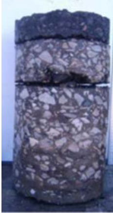
Figure 1: Hwy 400 Core exhibiting de-bonding in the surface and lower layers. Pre-design investigative core, Highway 400; McIntosh Perry, Hwy 400 Southbound)
