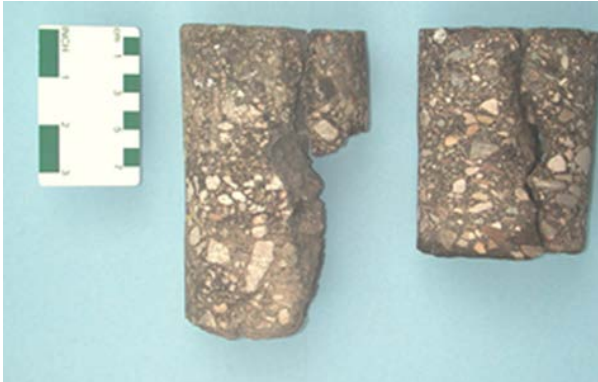
Figure 2: Hwy 10 cores showing full-depth cracking (Golder Associates, 2004) (Hwy 10, pre-design cores; Golder Associates 2004)
